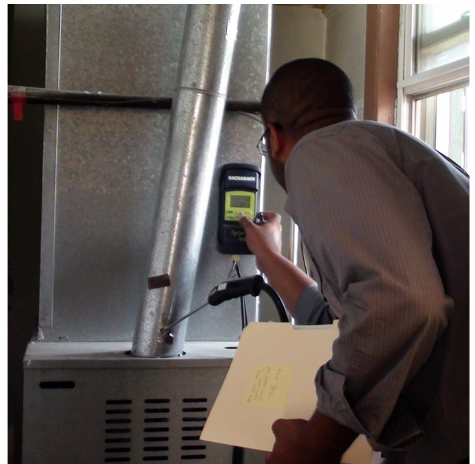
A member of the Energy Savers team conducts a combustion test on a furnace
